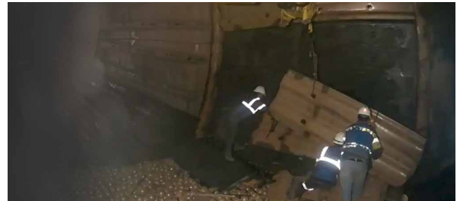
BEFORE: Crew exposed to multiple hazards during manual liner slinging
